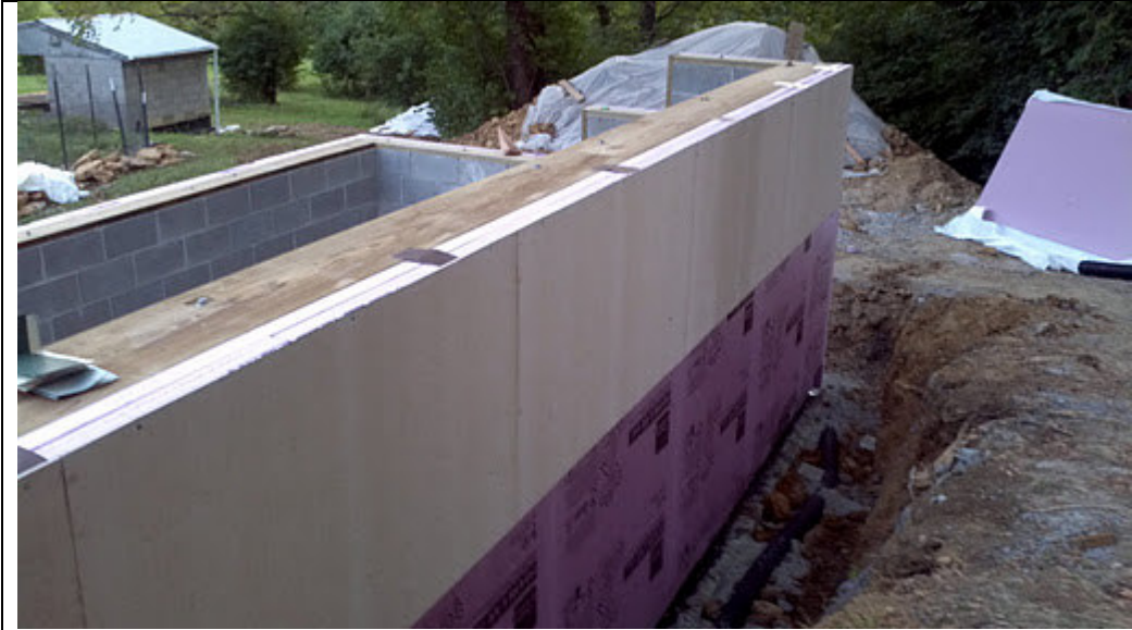
Insulation is on the outside of the walls so that the blocks can be a heat sink.
