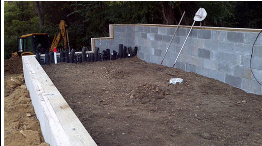
The top soil in place; note the 24 pipes exiting at the west end.
