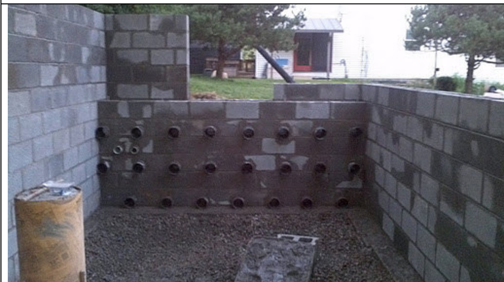
Note the 24 connectors into the plenum for the 24 perforated 4" pipes of the heat sink.
