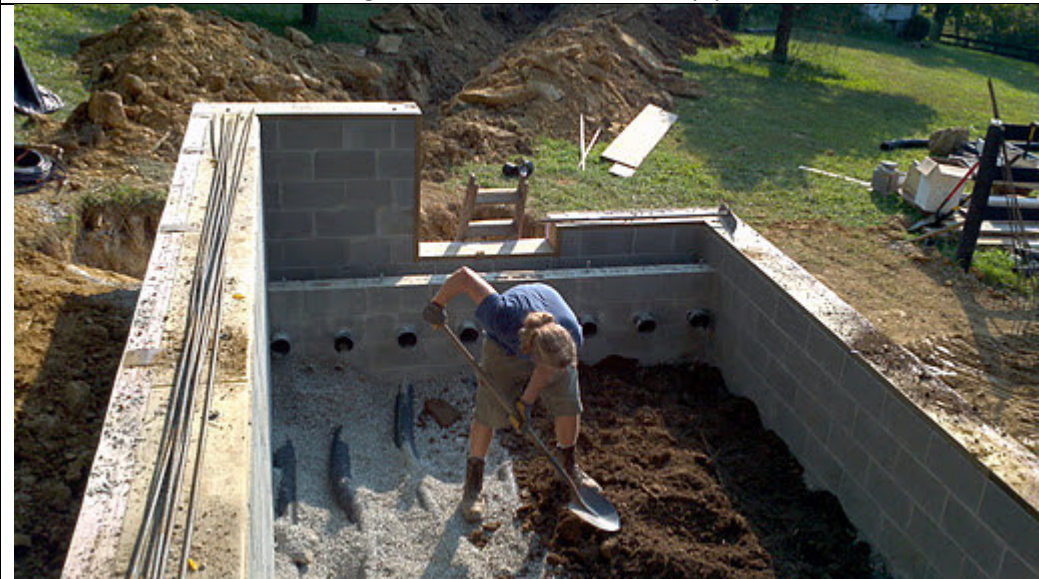
Last two rows of heat-sink pipes have a layer of dirt between them instead of rocks.
